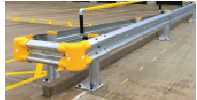
Service Yard - Edge Protection - HGV Safety Bollard
